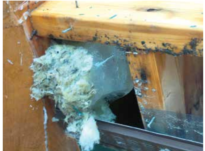
Solid block of ice build up in the soffit.
